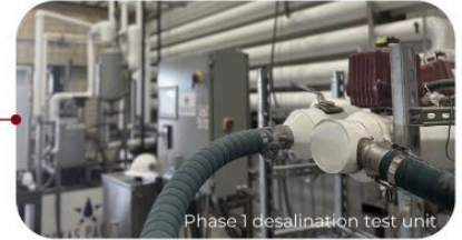
Phase 1 desalination test unit
